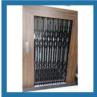
Collapsible Gate Goods Lift
